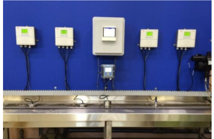
Standard configuration for online monitoring equipment instrument bench at our facilities
